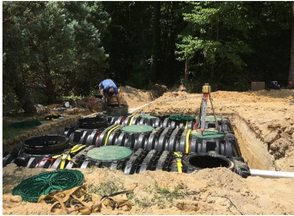
Underground Detention Tanks
